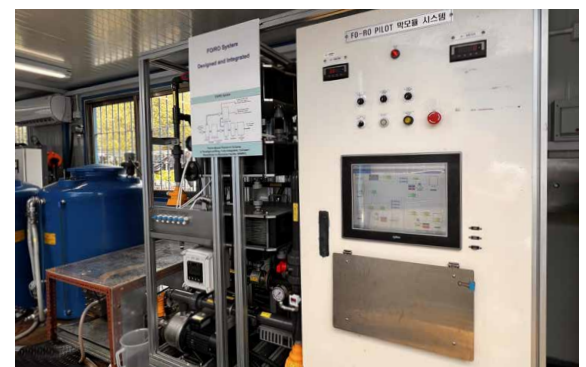
Pilot-scale hybrid forward osmosis and reverse osmosis system for high-quality water production from wastewater 用於高品質水回用的正滲透-反滲透集成系統的中試示範
